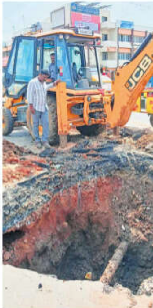
The cement pipeline, which is more than 50 years old, burst due to wear and tear and pressure variations | EXPRESS
