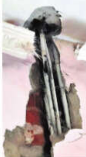
Part of the wall and ceiling collapsed after lightning strike | EXPRESS
